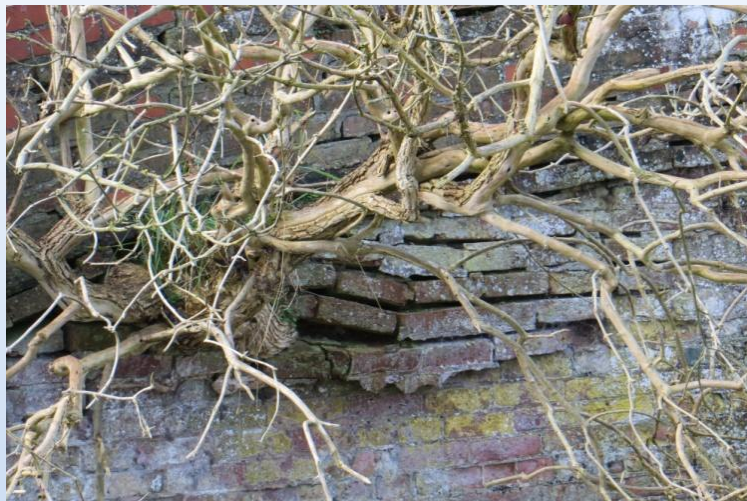
Tree bursting the brickwork of Eye Kettleby Lock Bridge
